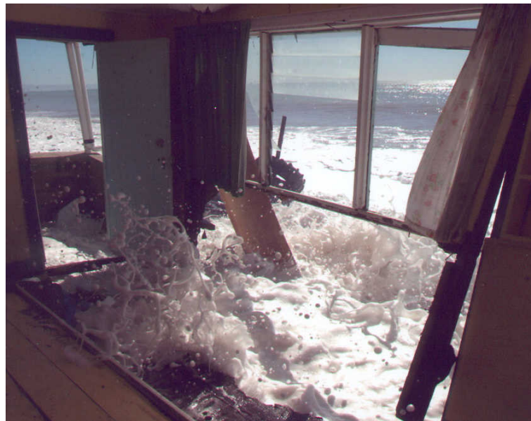
Figure A3.3: Damage caused to a coastal property at Haumoana (Hawke's Bay) by waves overtopping the gravel barrier in the Easter storm of 3–4 April 2002, assisted by high perigeon-spring tides. [Source: Hawkes Bay Regional Council].
