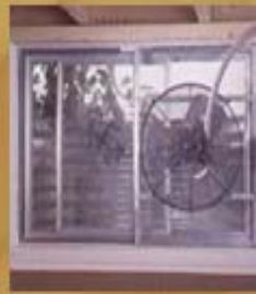
Turn off Window Fans
